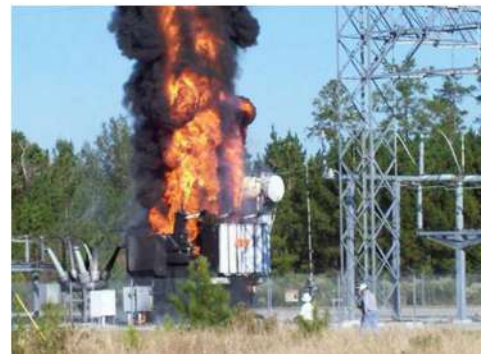
Fig. 1. Explosion of power transformer resulting from failures
